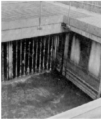
a. intake bar rack
